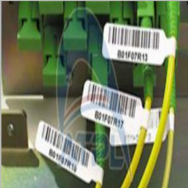
Wire and Cable Labels
