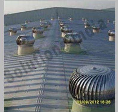
Self Rotary Ventilation Fans
