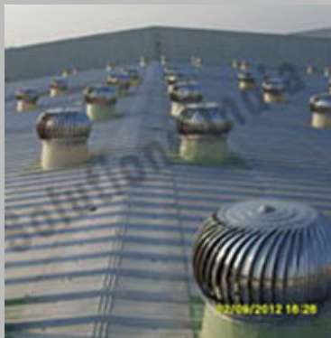
Rooftop Air Ventilator
