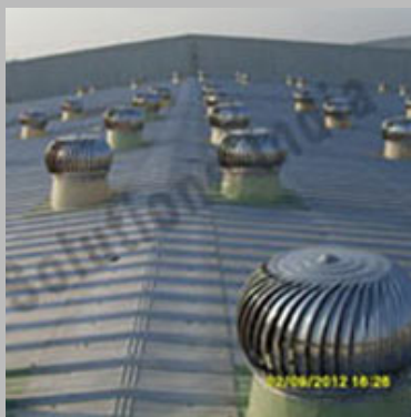
Rooftop Air Ventilator
