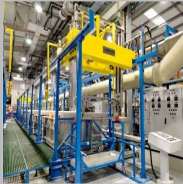
Fully Automatic Electroplating Plant
