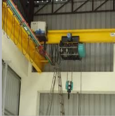
Overhead crane control equipments
