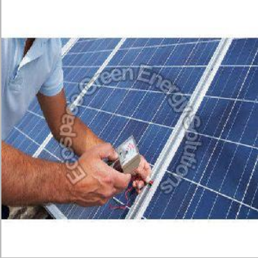
Solar PV System Maintenance Service
