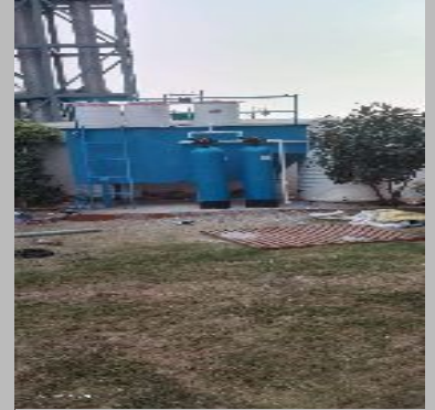
Containerized Effluent Treatment Plant
