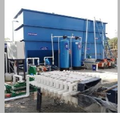
70 KLD Sewage Treatment Plant
