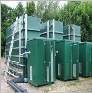
modular sewage treatment plant
