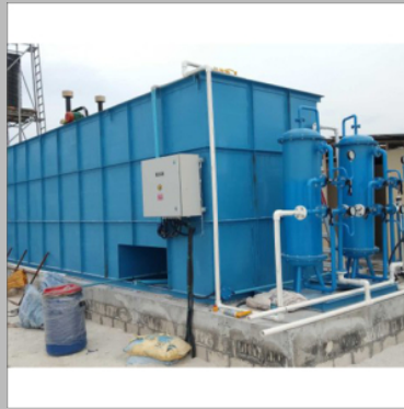
Portable Sewage Treatment Plant
