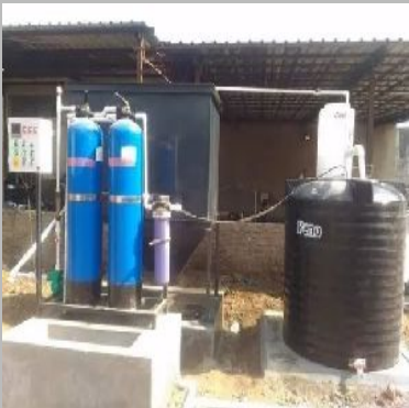
20 KLD Sewage Treatment Plant
