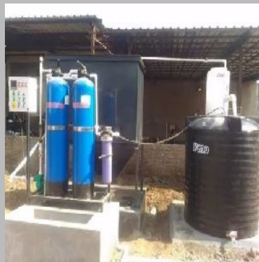
20 KLD Sewage Treatment Plant
