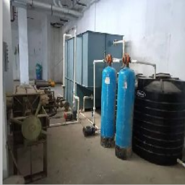
50 KLD Sewage Treatment Plant
