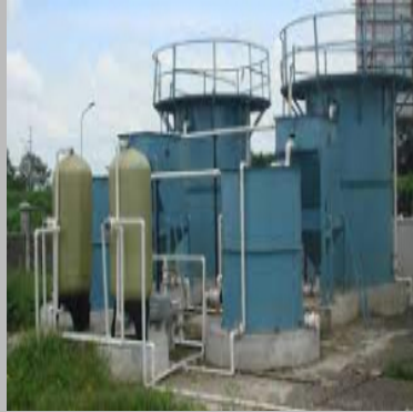
effluent waste water treatment plant
