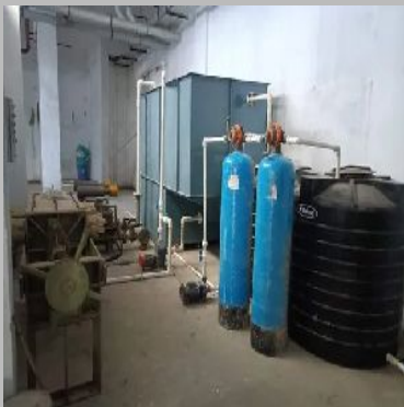
50 KLD Sewage Treatment Plant
