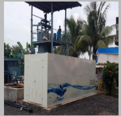
Containerized Sewage Treatment Plant
