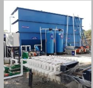
70 KLD Sewage Treatment Plant
