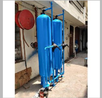
Iron Removal Plant
