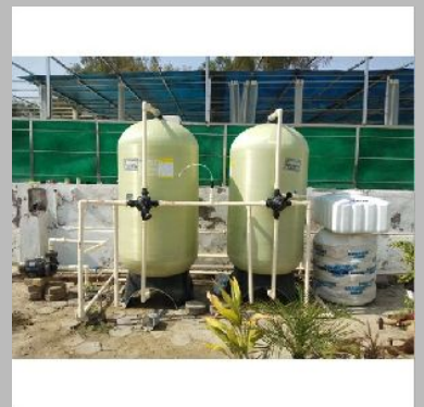
Water Softener Plant
