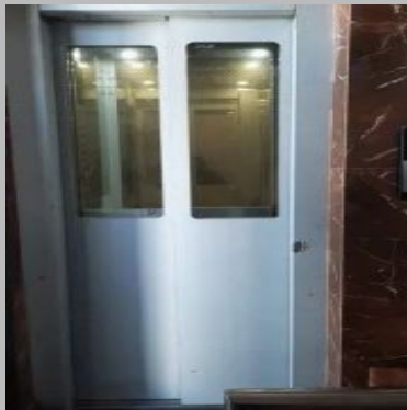
Automatic Hydraulic Elevator
