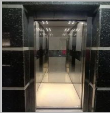
Automatic Passenger Elevator
