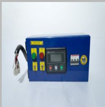
62.5 KVA Genset Control Panel
