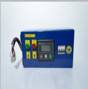
100 KVA Genset Control Panel
