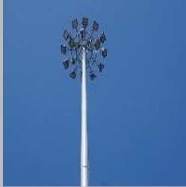
High Mast Pole
