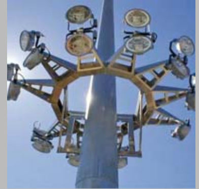
High Mast Lighting Pole
