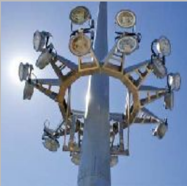
high mast light tower
