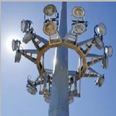
high mast light tower
