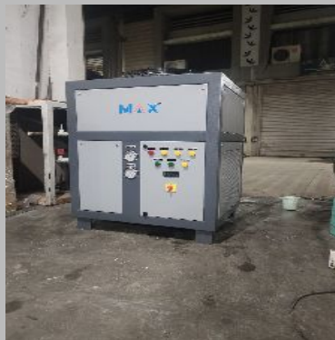
Hydraulic Oil Chiller
