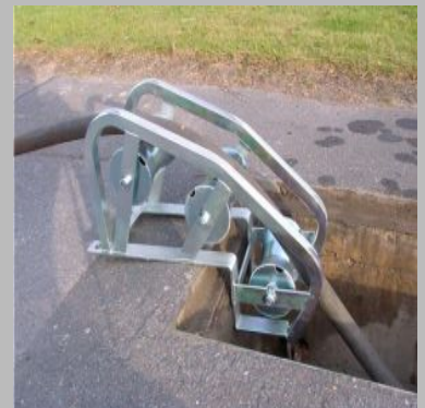
Manhole Cable Roller
