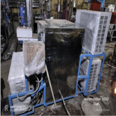
3000 Litre Water Chiller
