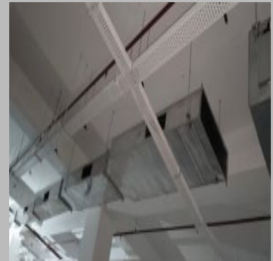
HVAC Ducting Service
