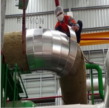
Hot Insulation Service
