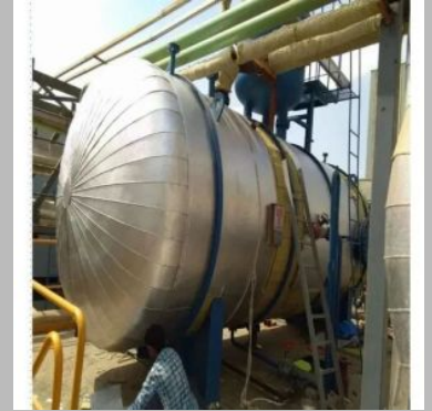
Cold Insulation Service
