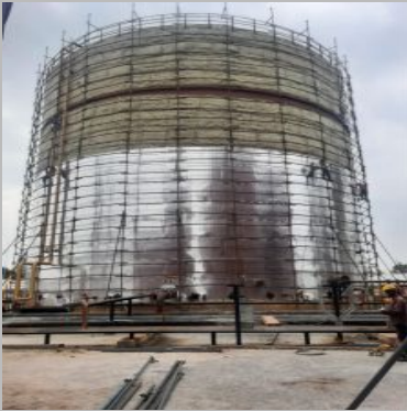
Acoustic Insulation Service
