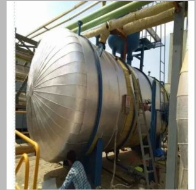
Cold Insulation Service
