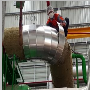
Hot Insulation Service
