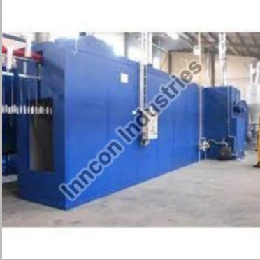
Powder Coating Plant
