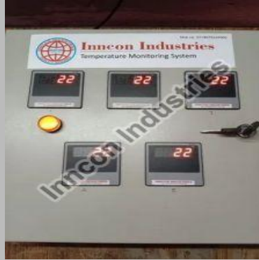
Temperature Monitoring System
