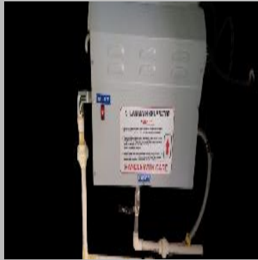
steam bath equipment
