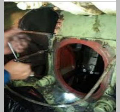
Cracked Engine Block Metal Stitching
