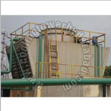
Timber Induced Draft Cooling Tower
