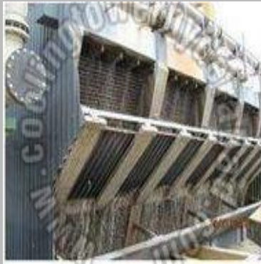
RCC Cooling Tower
