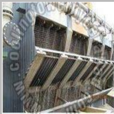
RCC Cooling Tower
