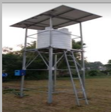
solar water pump system upto Installation
