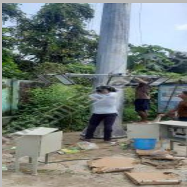
High Mast Light Pole
