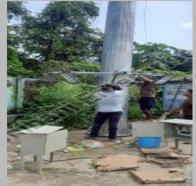
High Mast Light Pole
