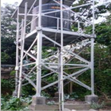
Water Pumping System
