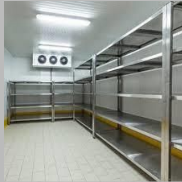
Vegetable Cold Storage Room
