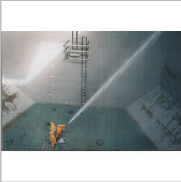
Tank Cleaning Chemicals
