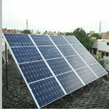
Residential On Grid Solar Power System
