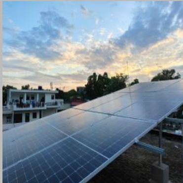
solar grid system
