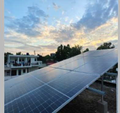
solar grid system
