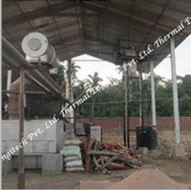
Industrial Hot Water Generator
