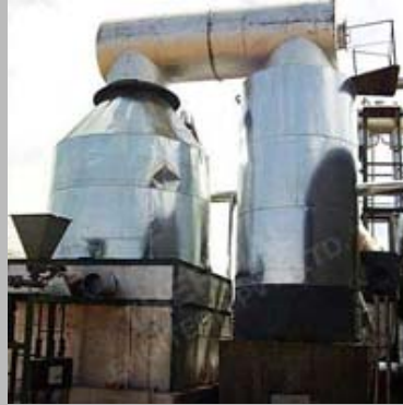
Hot Water Generators
