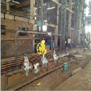
Indirect Heating Solution
