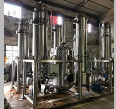
Falling Film Evaporator Plant
