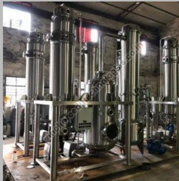
Falling Film Evaporator Plant
