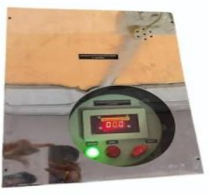
Earth Monitoring & Interlocking System with Hooter
