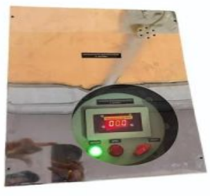
Earth Monitoring & Interlocking System with Hooter
